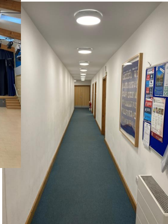
Installed energy-efficient lights
