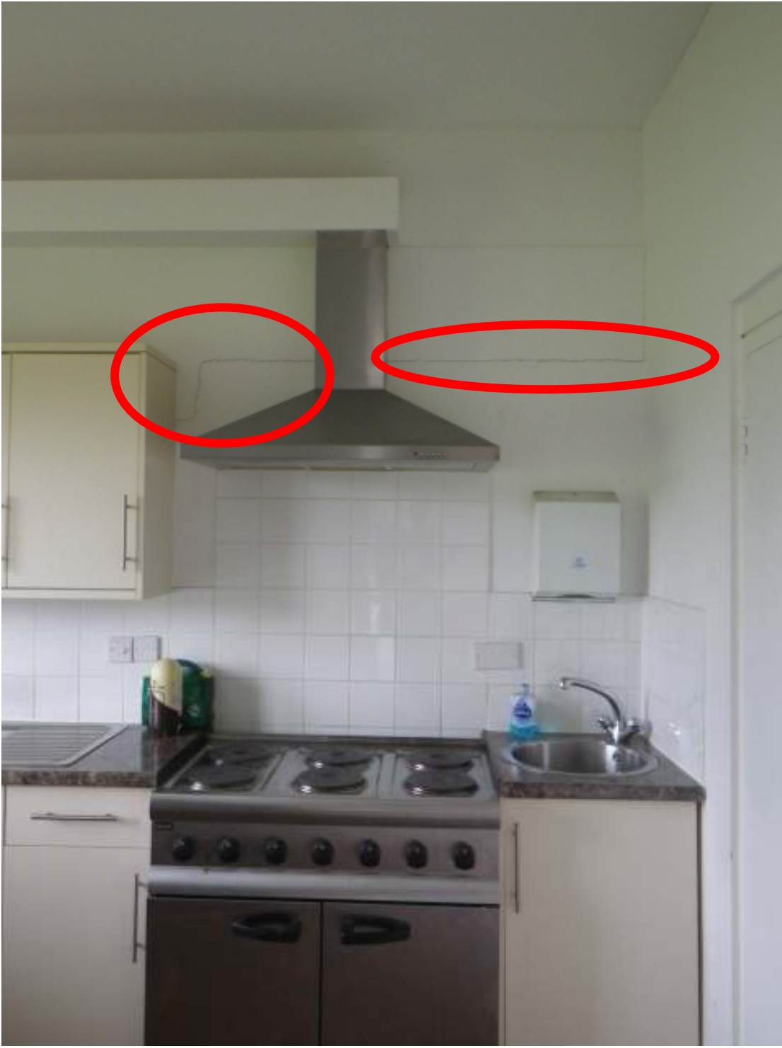
Cracking in kitchen
