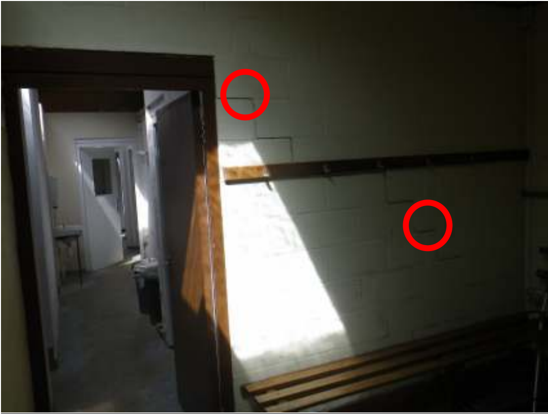
Changing area, diagonal cracking to walls
