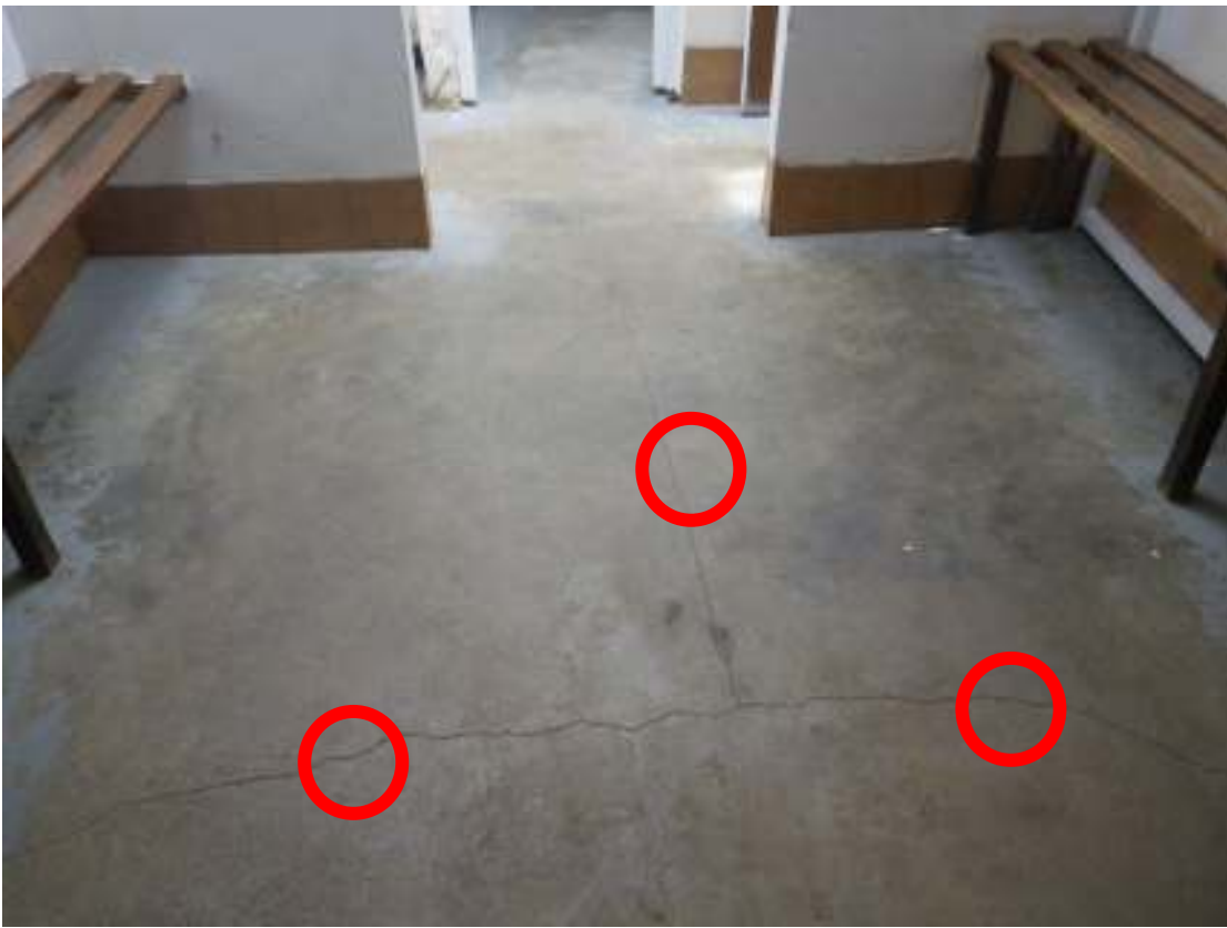
Changing 1, cracking to the floor slab
