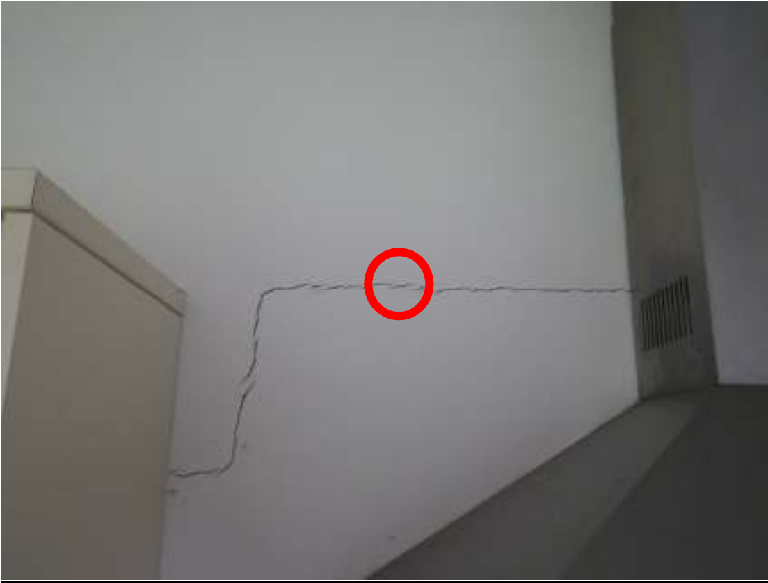
Kitchen, cracking to left hand side of cooker hood in previous photograph
