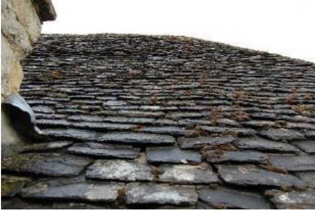
Photograph 7. Photograph showing the numerous naturally occurring gaps below the roof tiles.
