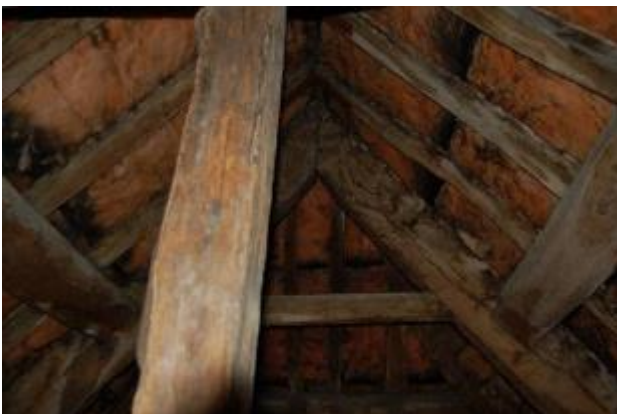
Photograph 5. A view inside the loft space. Taken from the east looking west.
