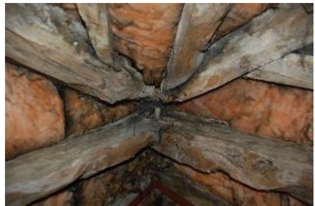
Photograph 6. Detail of the underside of the roof, which has been lined with fibreglass insulation, with bitumen and hessian roofing felt above.
